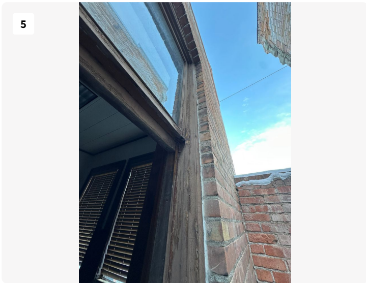
5 Detail current condition of windows.
