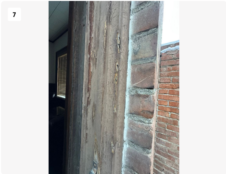
Detail current condition of windows.
