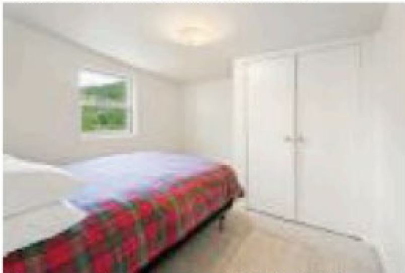
Here you can see the ceiling comes down below the door height.
