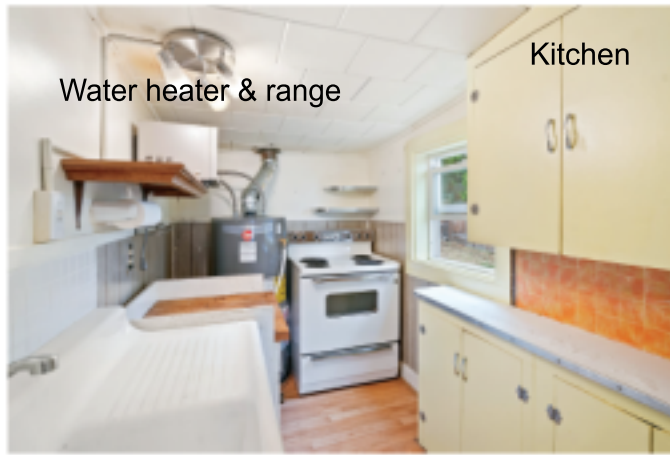
The electric stove burners are inches from the gas hot water tank. And the only counter space is 1' wide.
